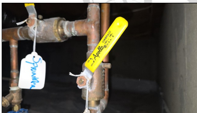
Secondary water shut off
