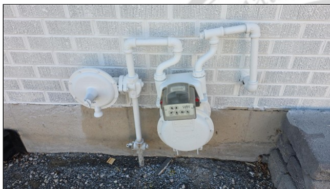
Gas meter and main shut off
